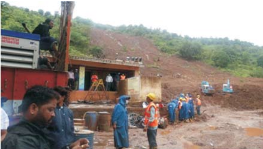
Figure 9: Site of landslide event at Malin village.
