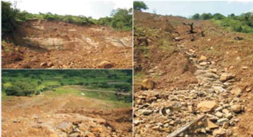
Figure 14: Nala along the slope poses instability and slope failure.
