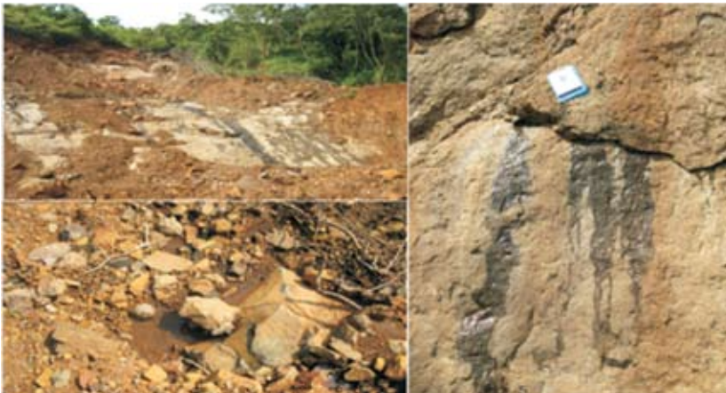
Figure 15: Seepage of water through rock poses instability and slope failure.
