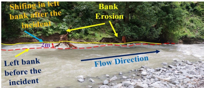
Photo 6. Collateral damage to the opposite bank (left) of Nanth Nala due to erosion.
