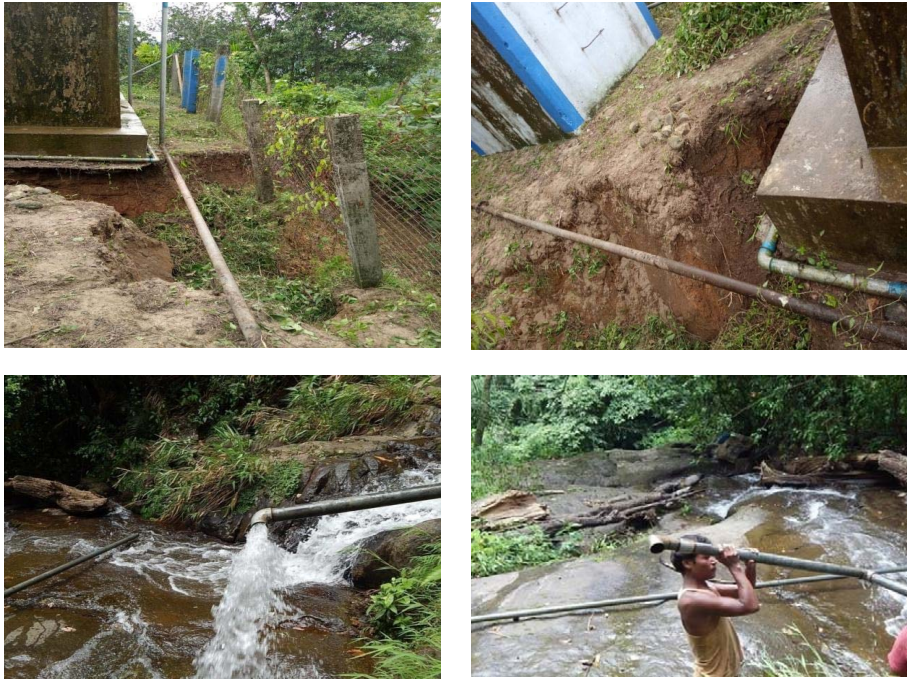
Fig 1D: Specimen photographs of eroded section of gravity main pipe lines (Sources: DDMA, SWKH).
