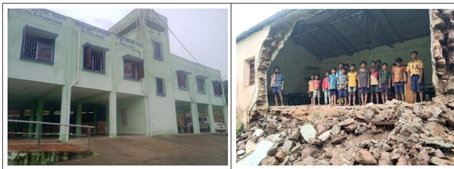
Fig-3: Hostel Block of UGHS (Upper Gradation High School) and the collapsed wall in Gangabada Village
