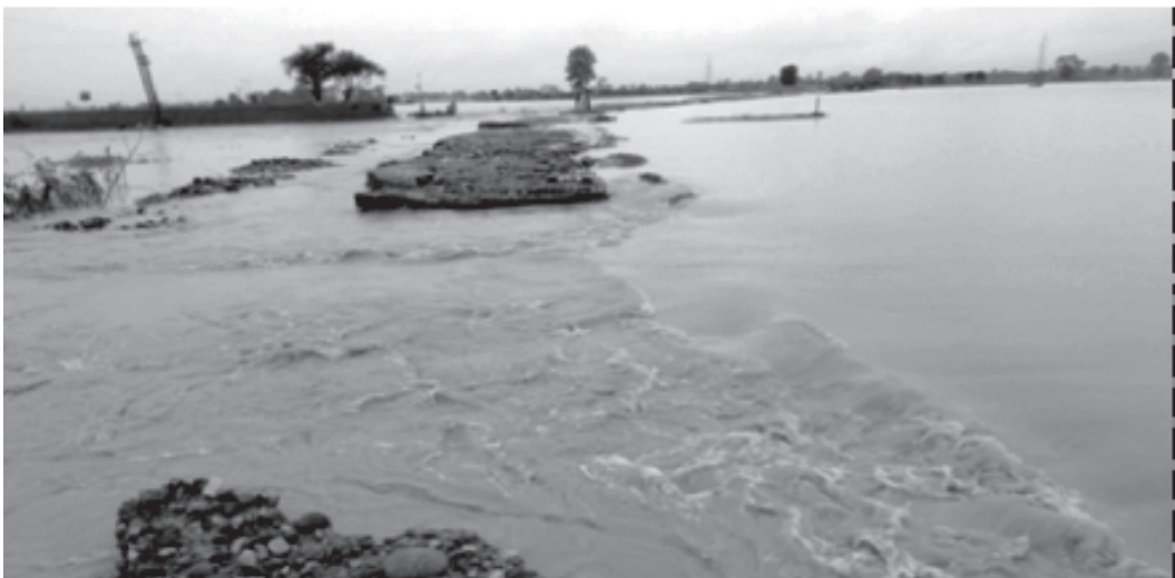
Figure 5: NH 52 After Floods
